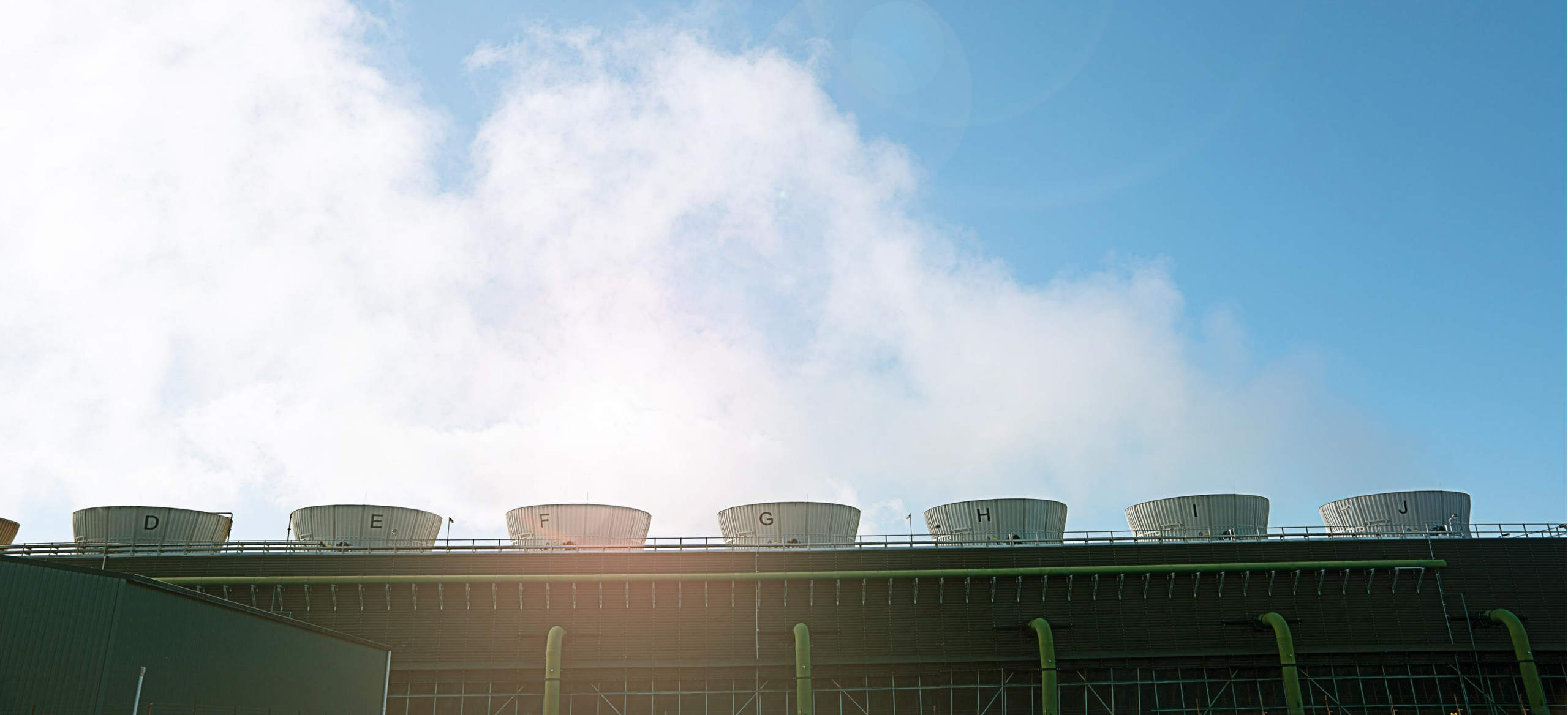
Ngā Awa Pūrua cooling tower
